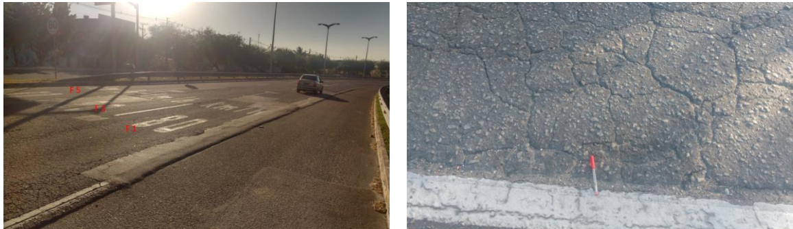
Figure 7 Defects observed in segments of Highway CE-501
